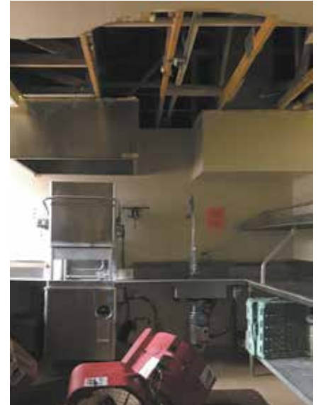
Damage above the kitchen sink
